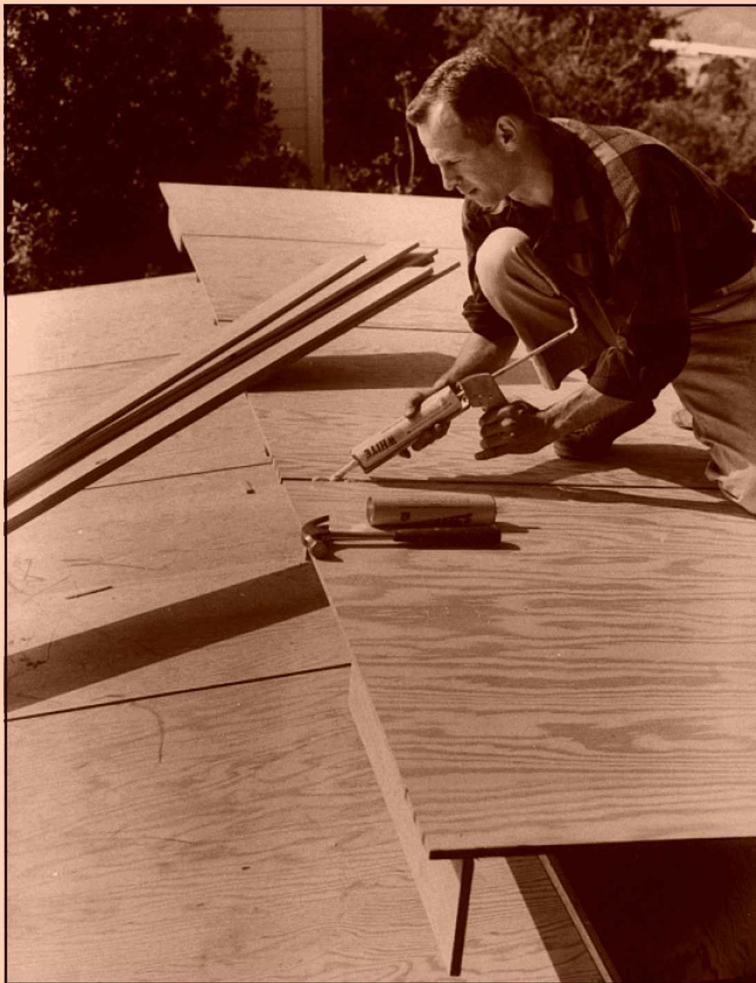
A man assembles a 'Do-it-Yourself' shed designed by architect Robert Anshen c1950
